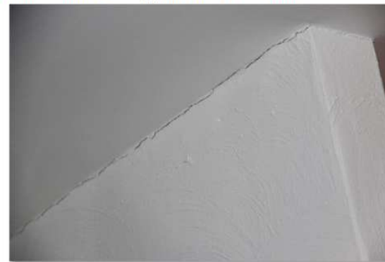
Figure 33 A2dr-cloison de la cuisine, fissuration des joints
